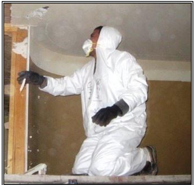
Photo 5: During demolition, workers should wear a minimum of goggles, gloves, and an N-95 respirator for protective gear. The worker above lacks eye protection and is improperly wearing his respirator straps.
