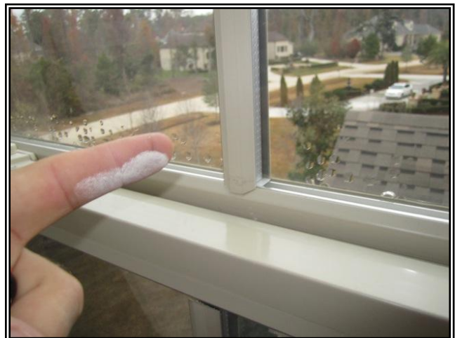
Photo 7: Inspector identifies visible dust after attempted cleanup. The presence of dust indicates that additional work is required.
