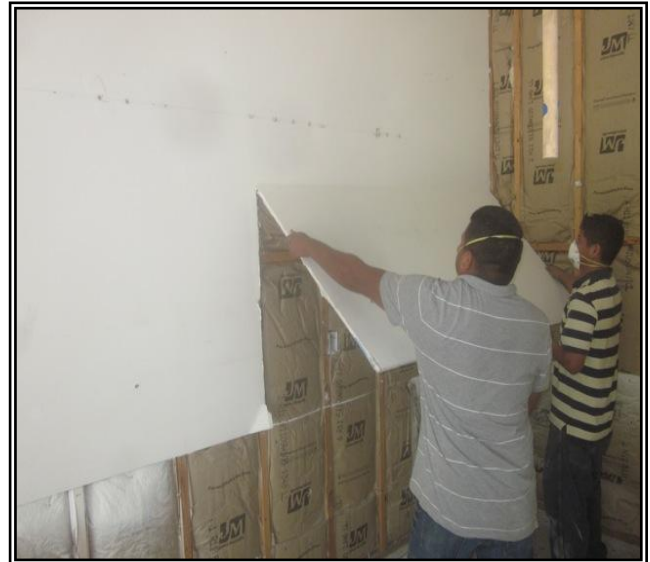
Photo 4: Most CDW remediation projects replace all drywall, but selective removal can be considered in some cases. Note that the workers are improperly wearing their respirator straps and the workers' street clothes are exposed to contaminated dust. This can be avoided by properly wearing a respirator mask and protective coveralls.
