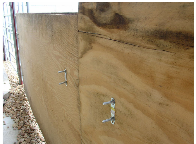
Figure 20. Protruding screws inside cattle handling paths could cause injury.
