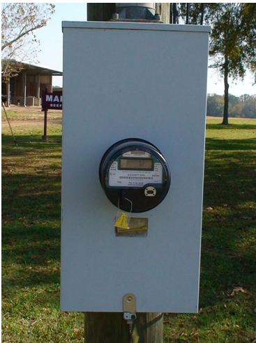
Figure 15. Electric and water utilities.
