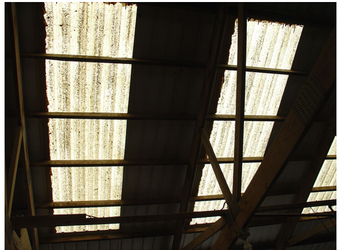
Figure 19. Translucent roof panels (skylights).
